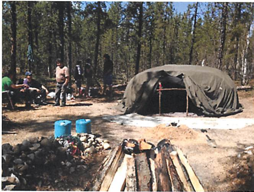
Figure 4. Students construct a sweat lodge during sikwan mamawewin under the guidance of Elders and traditional knowledge keepers.
